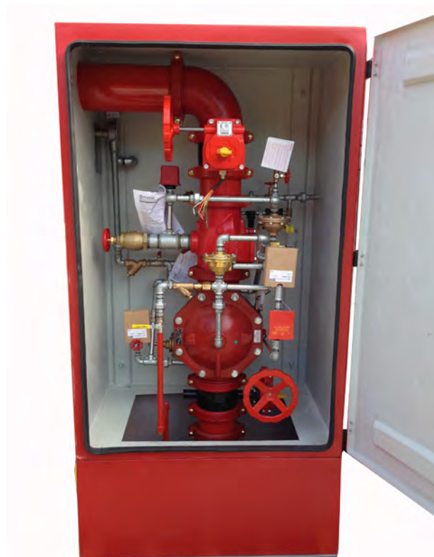
DELUGE PREACTION SPRINKLER
